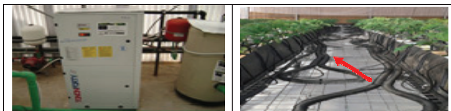
Photo: 3. Heat pump
