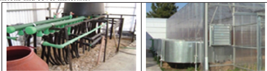
Photo: 1. The ground heat exchangers Photo: 2. The air dehumidification system
